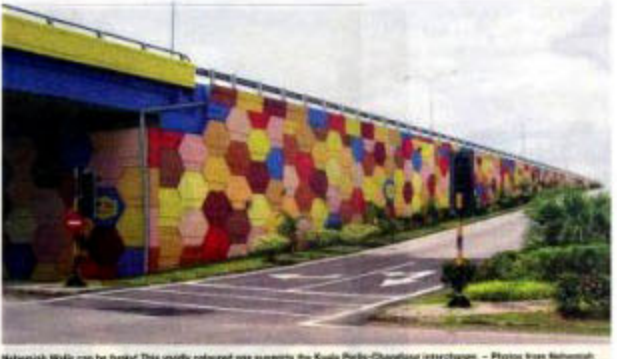
Nehemiah Walls can be funky! This vividly coloured one supports the Kuala Perlis-Changlun interchange. - Photos from Nehemiah Reinforced Soil Sdn Bhd
